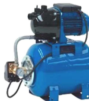
Fig 9: pressure switch system with pressure switch to replace with transducer
