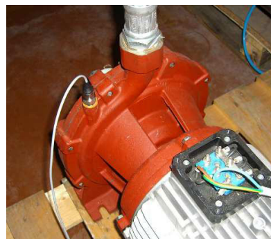
Fig 5: example of priming hole of pump delivery with transducer mounted
