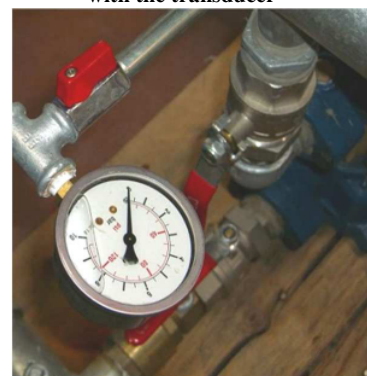
Fig. 7: Pressure gauge to replace
